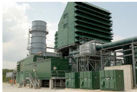
Gas-fired Combustion Turbine Generator Sewell Creek Energy Facility – Oglethorpe Power
