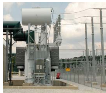
13.8kV – 230kV Step-Up Transformer
