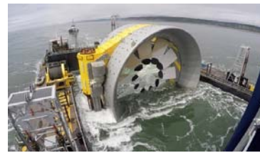
2MW OpenHydro tidal turbine installed in Canada in July 2018
