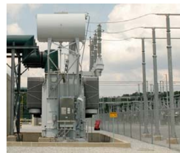
13.8kV – 230kV Step-Up Transformer
